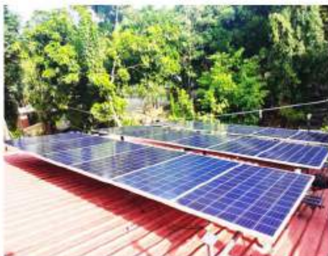
Existing Plant 6 KW
