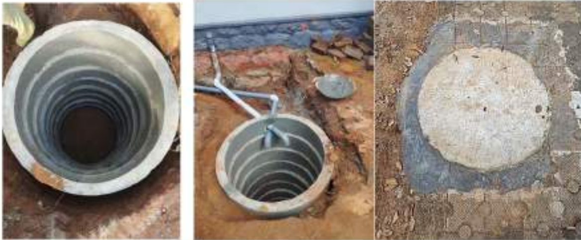
The new well for rain water harvest and two pits for rain water collection and Recharging in the church campus.
